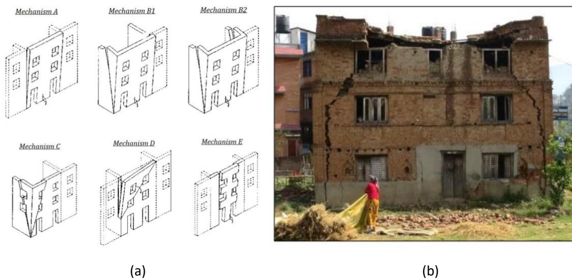
Figure 15. (a) Schematics of different overturning mechanisms (D'Ayala & Speranza, 2003); (b) Initiation of partial overturning of the façade of masonry building (Dizhur et al., 2016)
