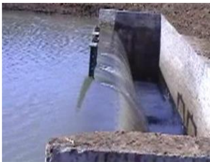
Figure 72. Night Storage Weirs
