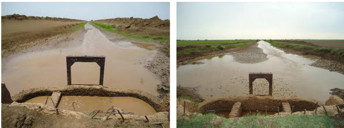
Figure 9. pictures of damaged and non functional NSW (Woldegebriel, 2011)
