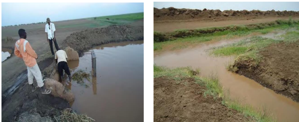
Figure 11. Right, farmers closing a NSW with Iron sheet, Left, Missing Field Outlet pipes (Woldegebriel, 2011).
