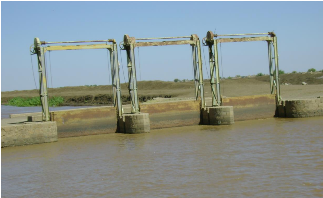
Figure 71. Sluice Gate Regulator
