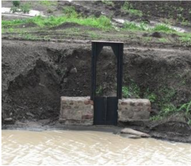
Figure 74. Field Outlet Pipes
