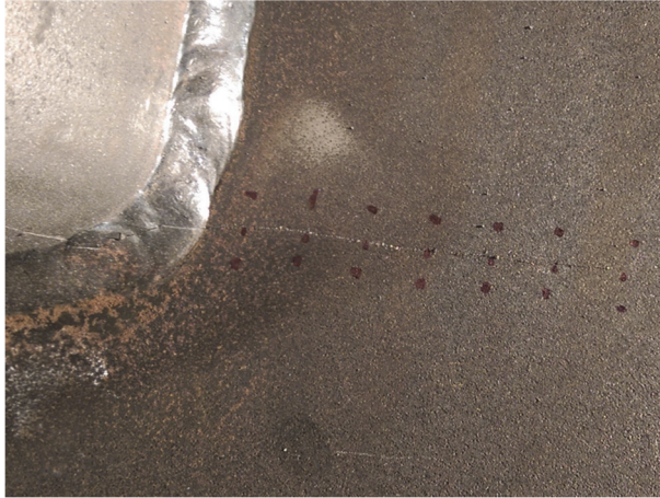
Figure 7.5: Close up photo of crack 1.
