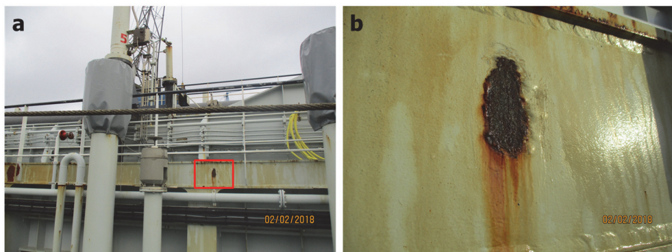
Figure 7.2: Location (a) and close up photo (b) of crack 1 on starboard side.
