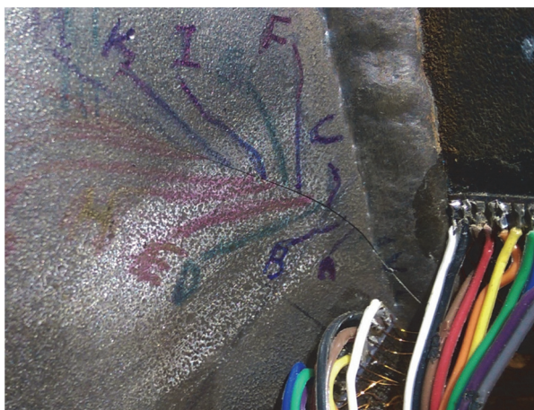
Figure 7.19: Close up photo of crack 3 in stage 6.
