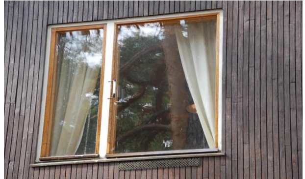
Figure 10: Simple and operable Vents contributes to wall breathability in the Helsinki House (photo: Alix Henry)
