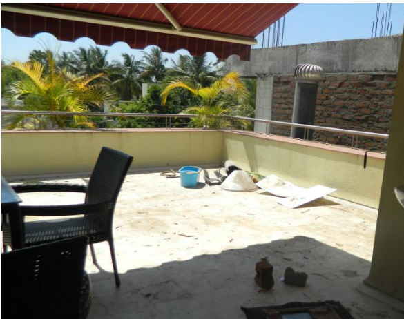
Figure 2: Top (a) Laying out of the TOD system during construction and below (b) the finished terrace slab with the TOD system within
