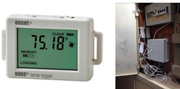
Figure 8: Electricity meter (right) and thermometer (left); Collecting data from the residential units
