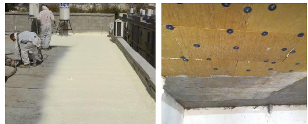
Figure 10: Insulating the elevated floor with rigid mineral wool boards (right) and polystyrene foam on the roof (left) of the Sderot building.
