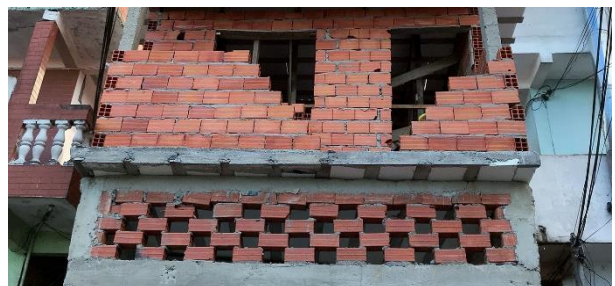
Figure 8: (Second outcome) Environmental DIY facades started spontaneously being built in Paraisópolis. Picture taken in April 2018.
