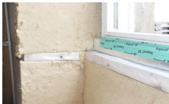
Figure 3: Internal wood-fibre insulation, which aims to provide active moisture control working in combination with the demand control mechanical ventilation system.
