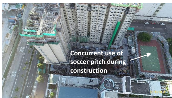
Figure 9: Construction of FTSW development with deferred closing of the existing public soccer pitch to minimize disturbance of its use by the community.
