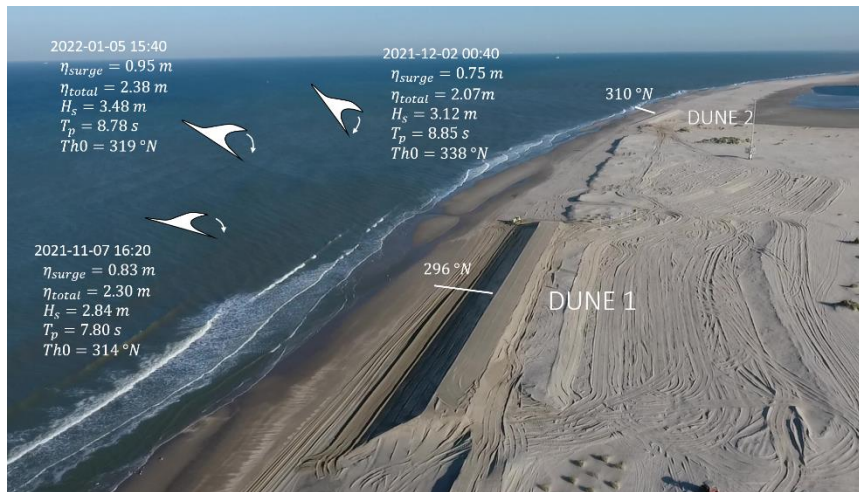
Fig. 1 Aerial photograph of the field site including offshore hydrodynamic conditions during the three campaign storms. The water levels were measured at the Hoek van Holland and Scheveningen stations. The wave conditions were measured at the offshore EuroPlatform station
