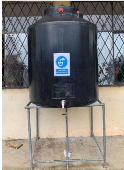
FIGURE 9: Final drinking water tank
