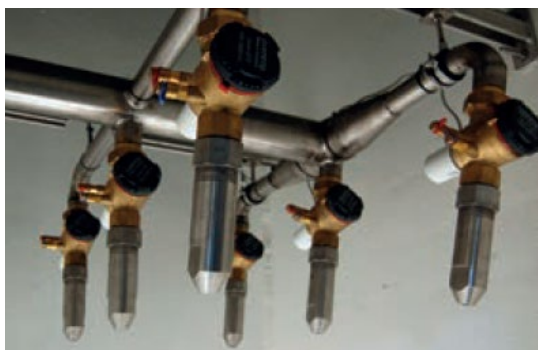
Figure 28 The 9 water spray heads of the Climate Cascade at The Four Elements hotel (Heirbaut, 2019)
