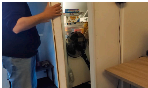
Fig. 2. Rudolph shows the sound insulation that reduces the noise from the ventilation system.
