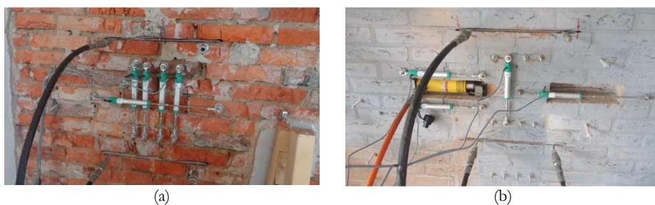
Figure 3.3: Semi-invasive in-situ tests performed by EUCentre on existing masonry: (a) double flat-jack test; (b) shove test. Photos were extracted from Graziotti et al. (2014).
