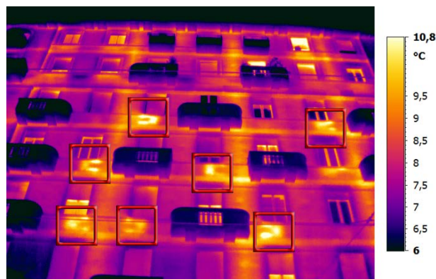
Figure 8 - Detail of the temperature distribution on the upper part of the façade (Case Study 2), above the main entrance. In the red squares, the warmer areas due to the heat flux generated by the heaters. The reduced thickness of the masonry where the heaters are located causes higher surface temperatures, especially at the connections between the heater and the hot water pipes.
