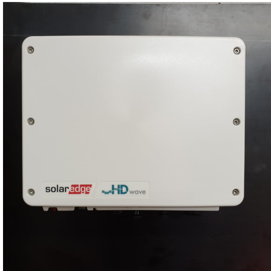
(a) Installed inverter.
