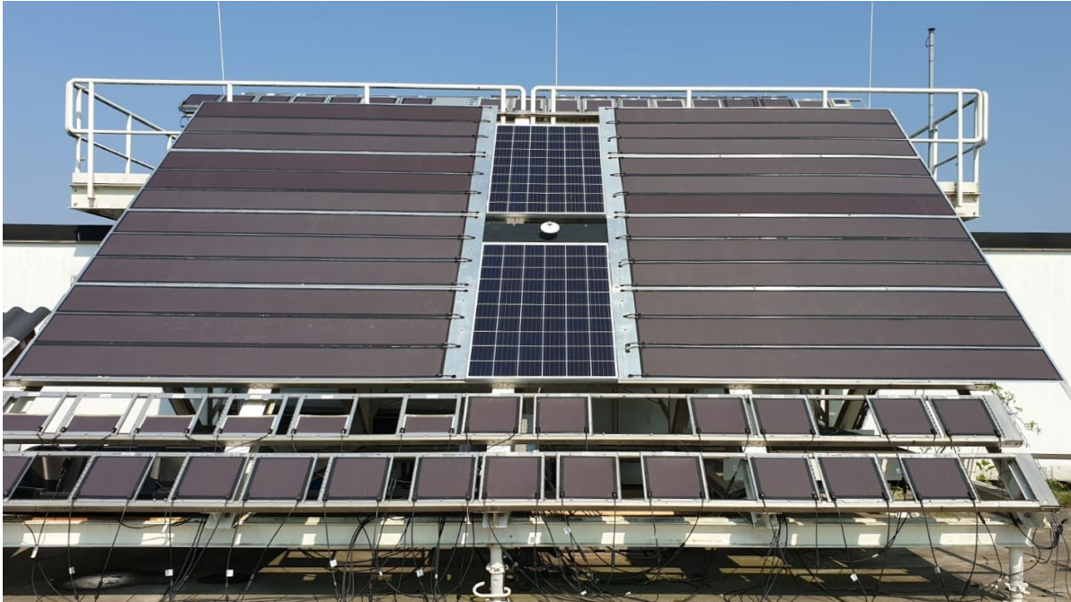
Figure 5.23 Completed performance monitoring system.
