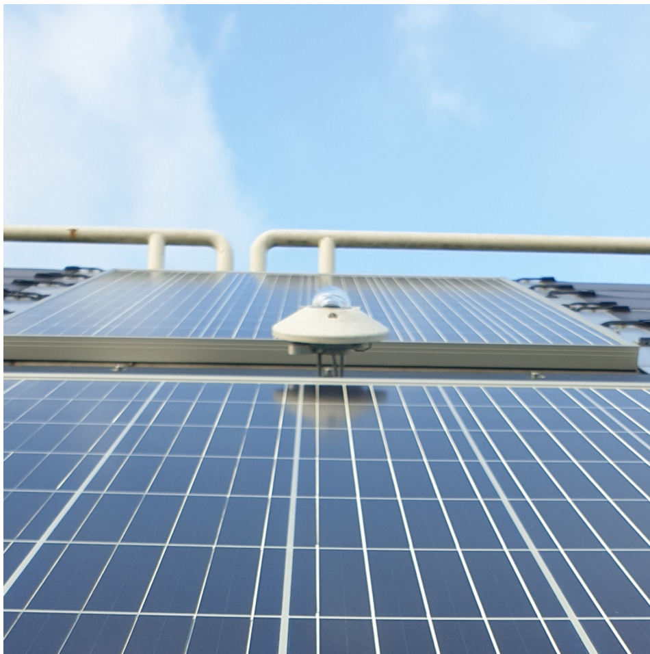
Figure 5.19 Kip & Zonen CM21 pyranometer mounted in the plane of the array to measure I_{POA} .
