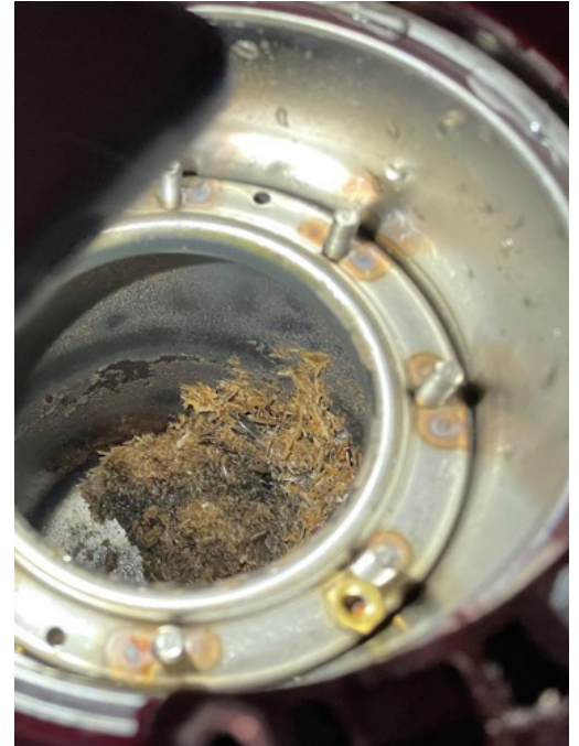
Figure 62. Limescale flakes within a Quooker reservoir
