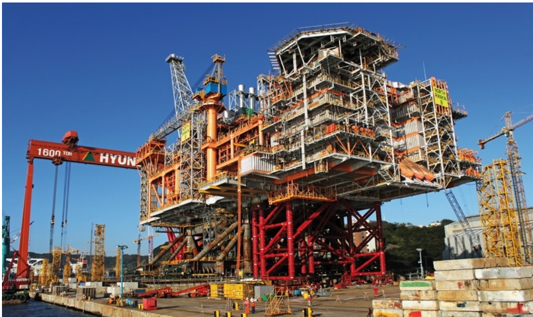
Figure 2.5: North Rankin B Topsides with DSF and Mammoet Jacking System JS2400 (courtesy Mammoet)
