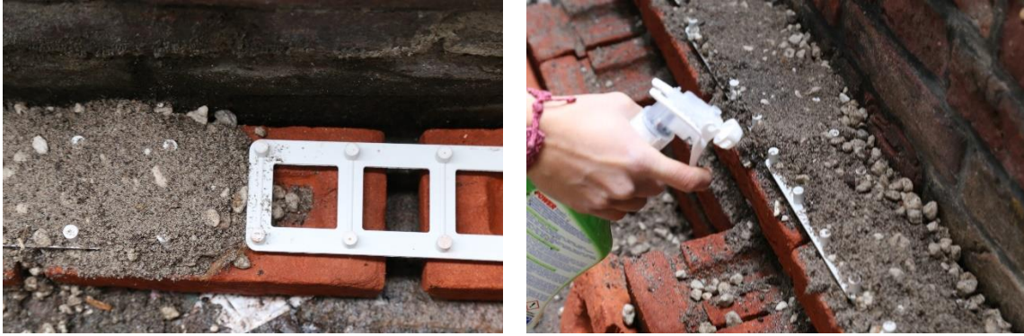
Figure 86: Assembling process of the wall with the TGS upper light substrate (own work)
