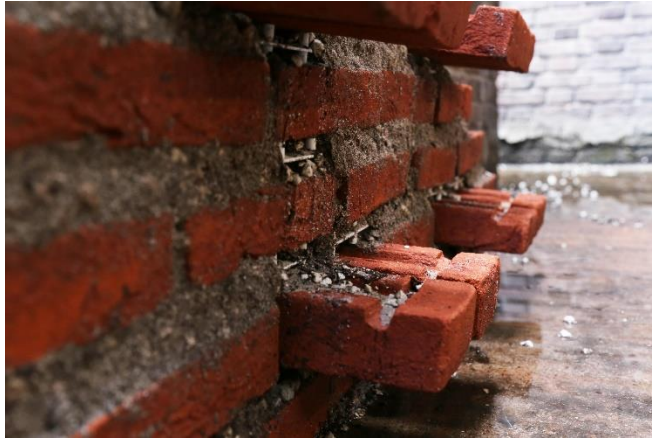
Figure 88: Erosion of the soil substrate after water pouring
