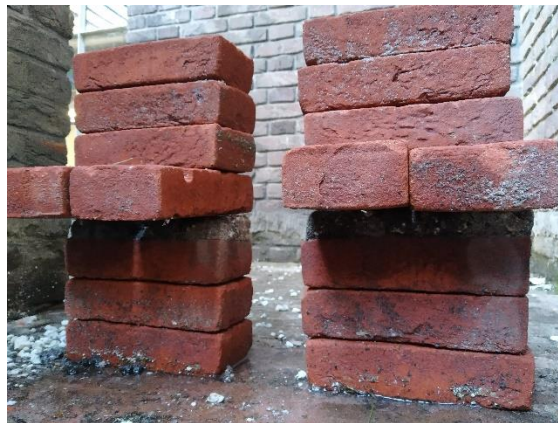
Figure 103: no wash-out after pouring water inside the frogs (own work)
