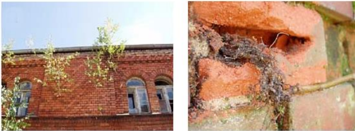
Figure 7: B pendula trees growing on the brick wall of 115-year old building, Roots growing in the air-bricks (Trocha, L. K. et al. 2007)
