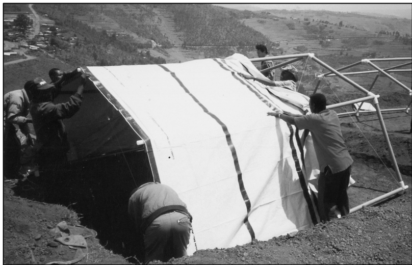
Figure 16-17. Rwanda Refugees assembling the Paper emergency shelters at Gihembe Refugee Camp, Rwanda, 1994 Source: Ban, "Paper Emergency Shelter," 112-123, 121-122.
