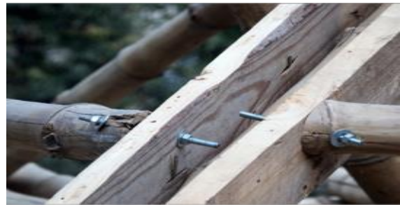
Figure 95: Insufficient structural connections
