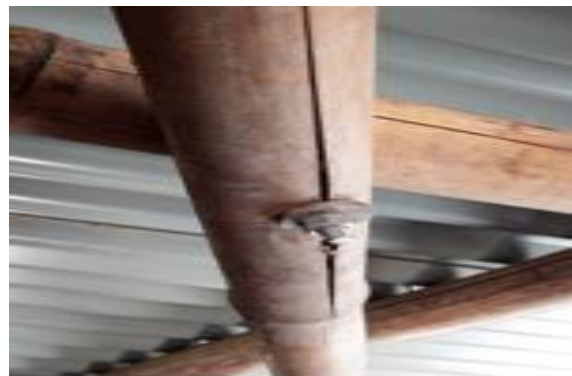
Figure 96: Insufficient structural connections
