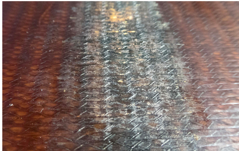
Figure 4.29: Degradation of the surface of the cyanate ester support plates after welding
