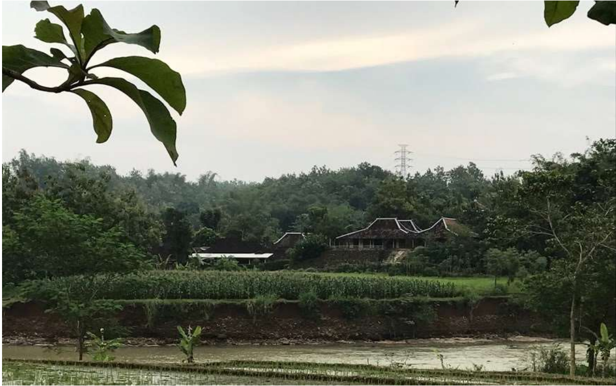
Figure 26 Poor river cliff condition in Keduang River (private documentation)
