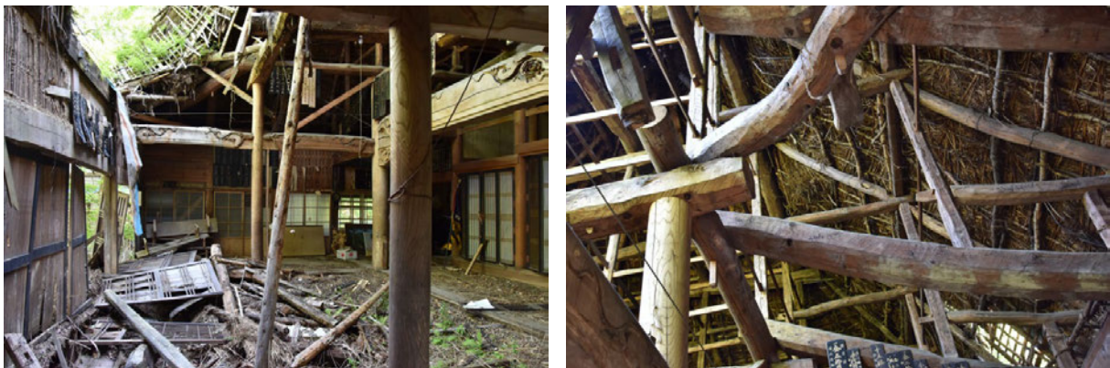
Figures 2, 3 Interiors, debris and roof structure within the temple. Storm damage is exacerbated by snow build-up during the winter months.
