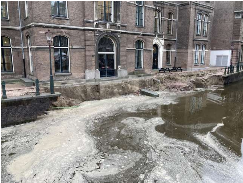
Figure 1.1: Collapsed Grimburgwal, Amsterdam [25].
