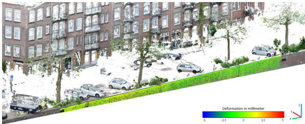
Figure 4.9: Point cloud with deformation points. The deformation points are coloured to the deformation in Y direction, which is the direction perpendicular to the quay wall. The position of the reference plates with control are indicated with an arrow.
