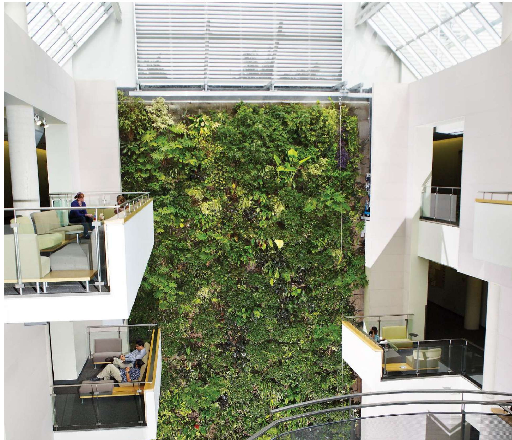
Figure 2. 18m tall - green wall installed at the University of Guelph-Humber, Canada. (Nedlaw Living Walls, 2004)
