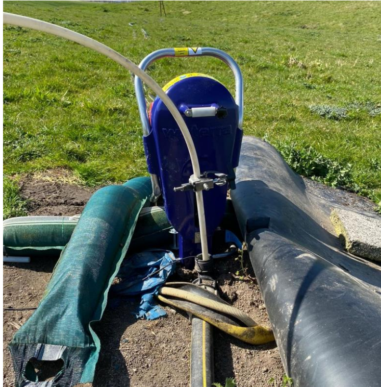
Figure 5.4: Jiggle pump installed in aeration well with mechanical driver
