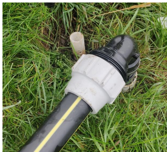
Figure 2.4: Opened aeration well and piping system leading to the divider
