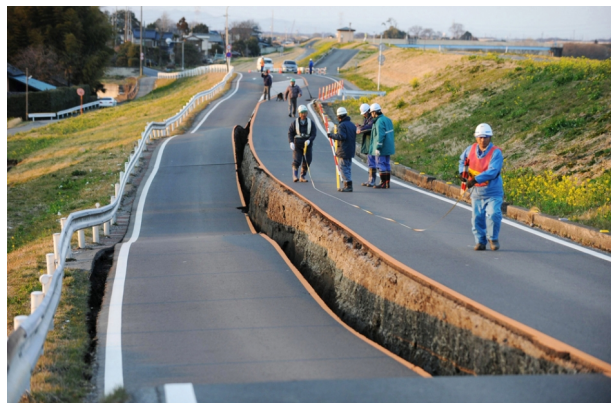
(b) Differential settlements in pavement and embankment structure
