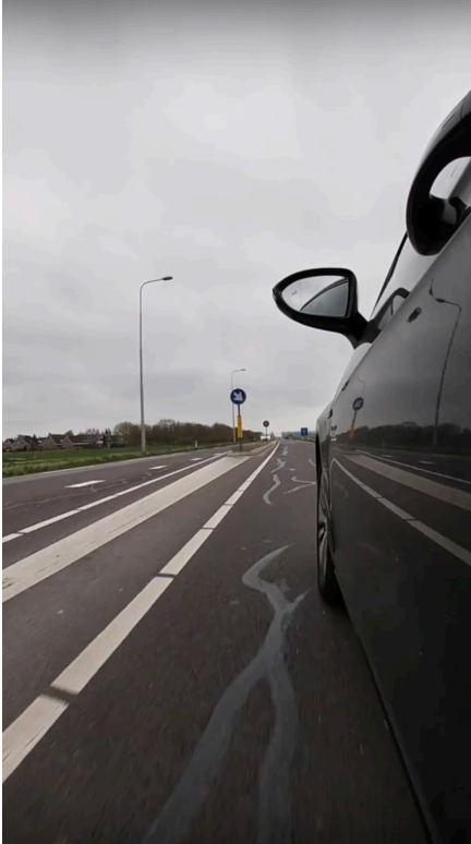
(b) Asphalt repair marks
