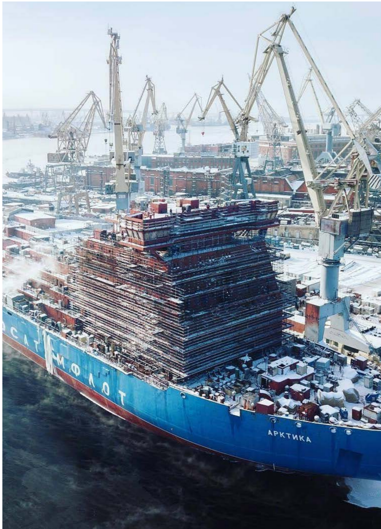
▼ photo/02 Nuclear icebreaker Arktika (LK-60Ya-class lead ship) under construction in St. Petersburg
