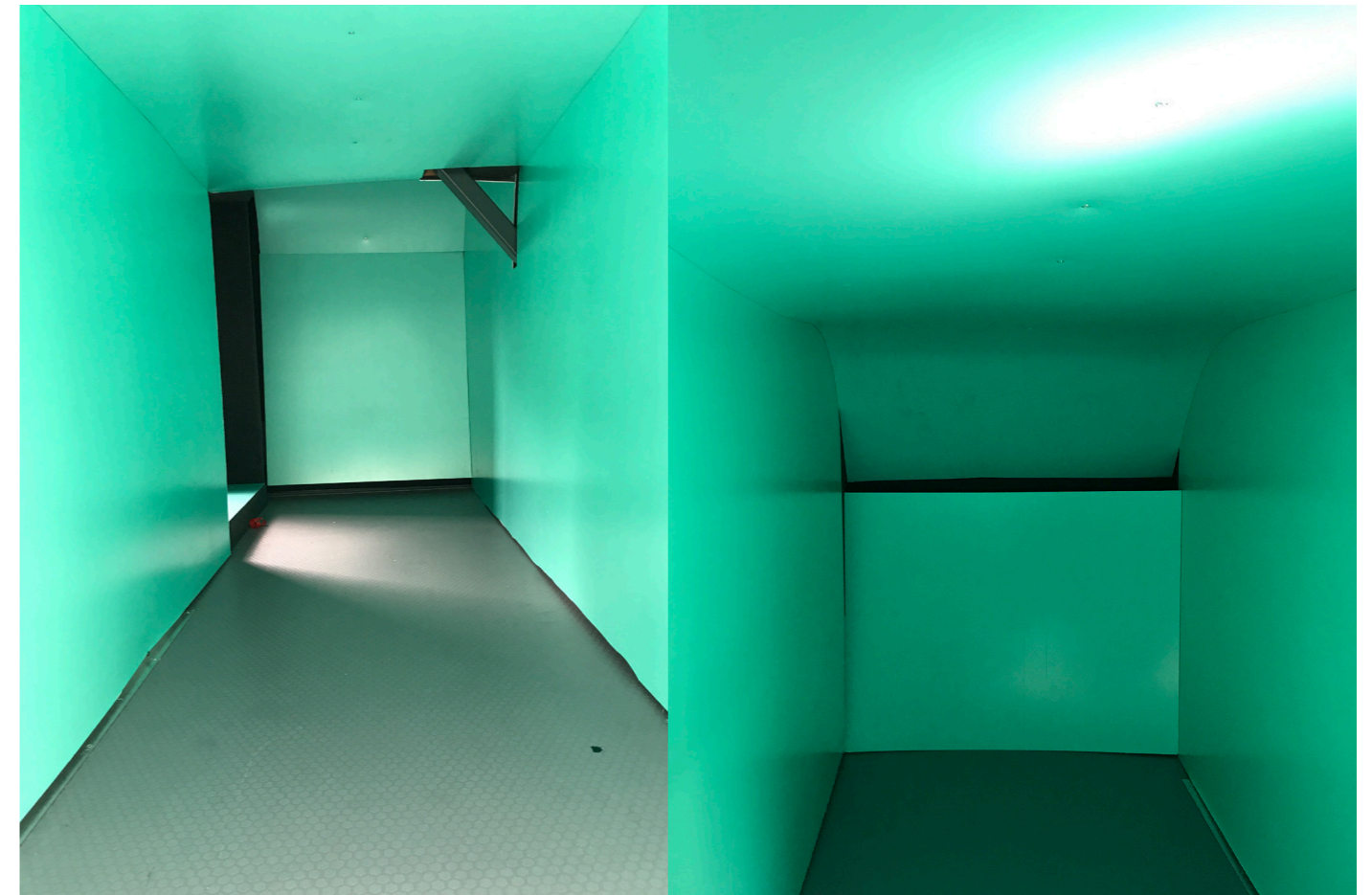
Most of the entrance has been covered with the first layer of transformation. The following steps were to finish it completely and to start with integrating the light and the lower ceiling. Before the light could be integrated, it was necessary to know how to do so. Several possibilities have been tested and for this mock up, the easiest and best way was to stick it on the already attached ceiling.
