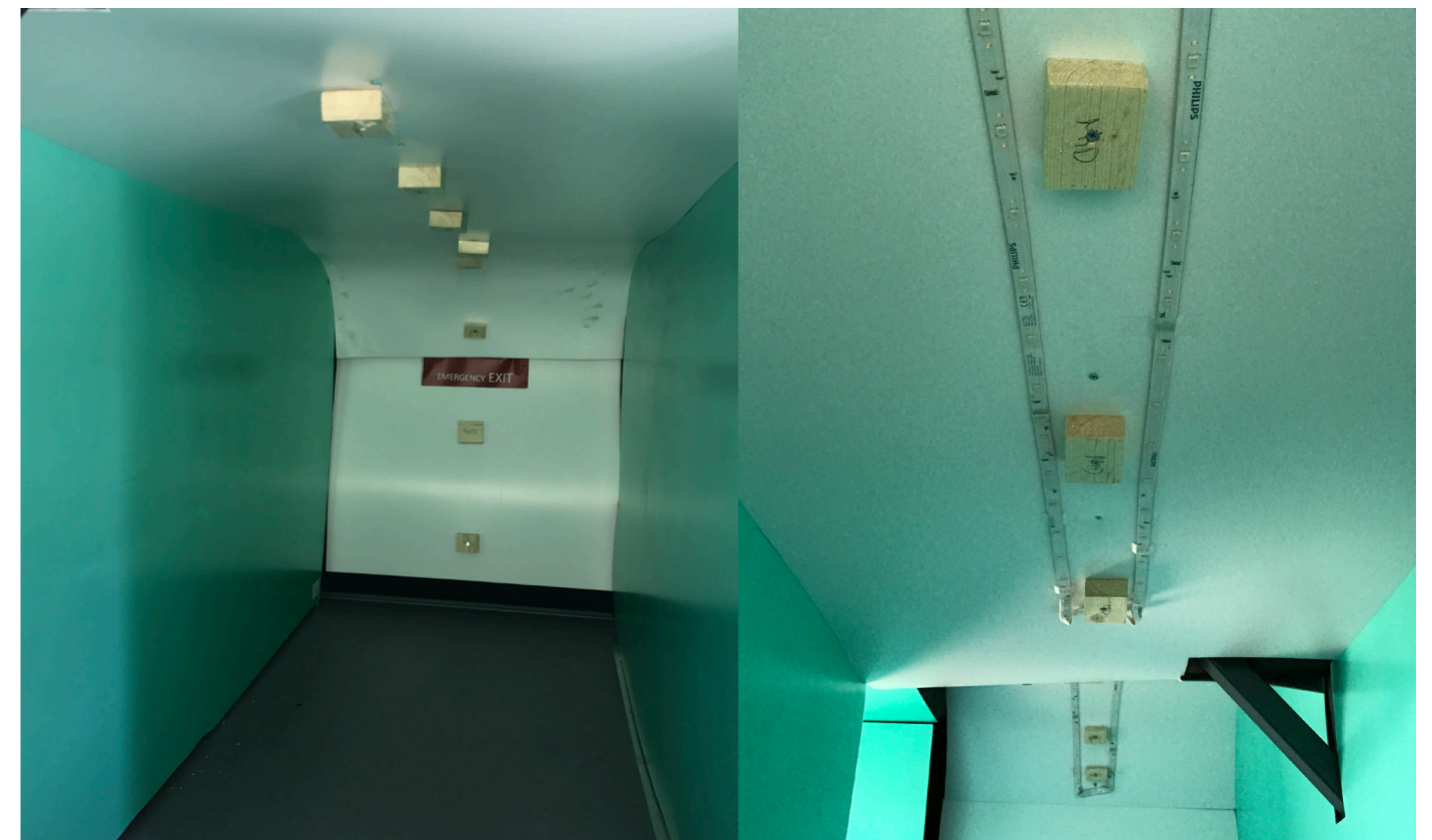
First, the protection foil needed to be removed, followed by attaching the attachment material for the lower ceiling as can be seen below. After that has been done, the LED strips have been attached with their self sticky side and with extra tape, just to be sure.
