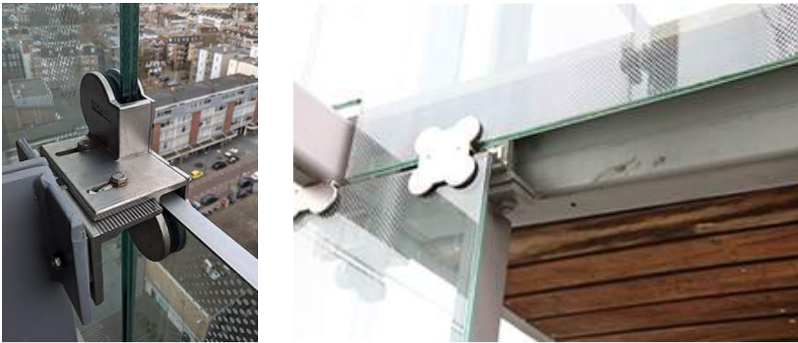
Fig. 4.6: Low friction clamp allowing movement in 3 directions, guardrails at de Karel Doorman , Rotterdam
