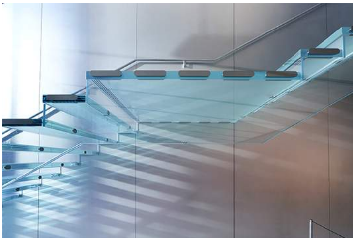
Fig. 4.8: Thick insert embedded connection at stair tread to balustrade, Apple San Francisco (seele, 2016)
