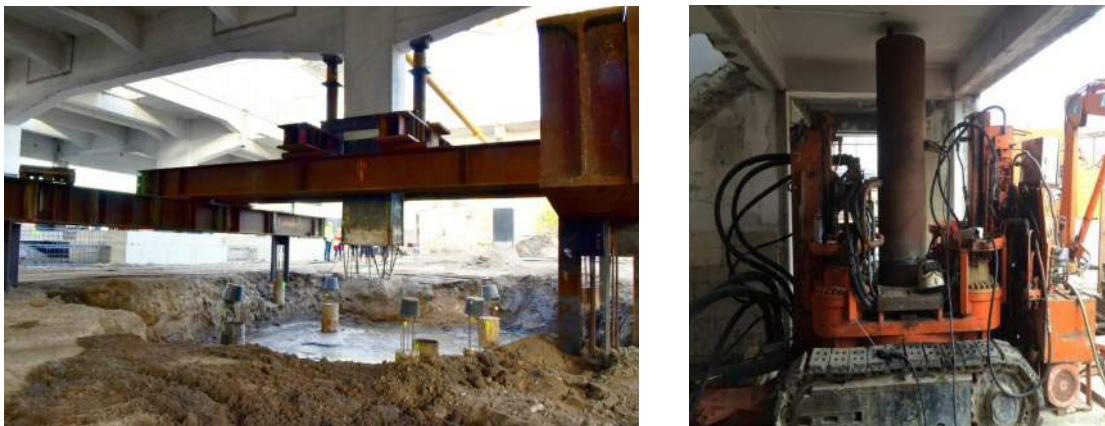
Fig. 5.6: Left: Shoring frame at column base. Right: Piles driven at interior columns. (Courtesy: ABT)
