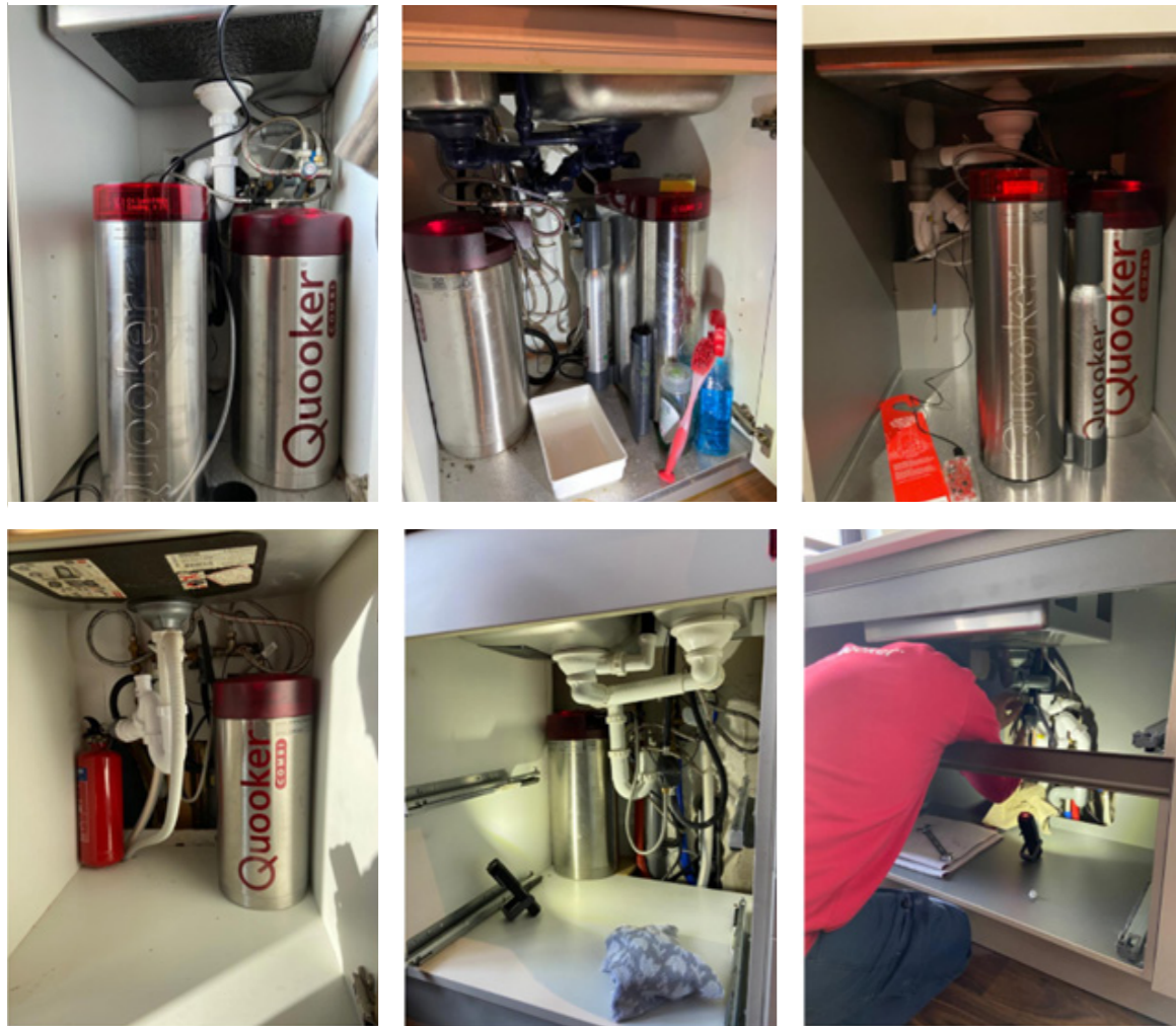
(Figure 13: different compositions of Quooker systems in kitchen cabinets under sink during an observation day with a service technician)
