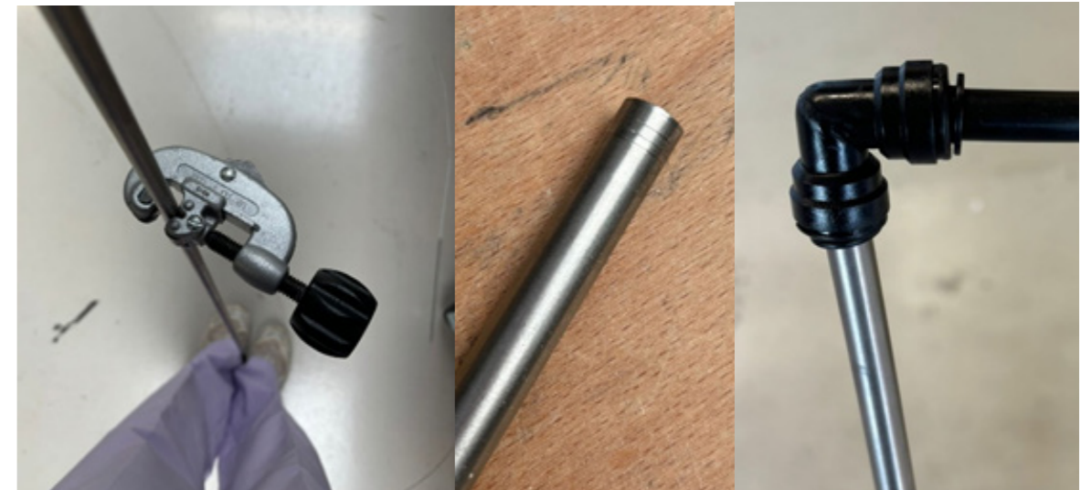
cold water inlet and outlet pipes were cut into the desired length of 115mm for the inlet and 415 mm for the outlet pipe. Then, creating a scratch on the outer surface of the stainless steel pipes so that the push-in fitting is securely attached to the pipes. On the other side of the push-in fittings, 10 mm LLDPE flexible pipes are attached.
