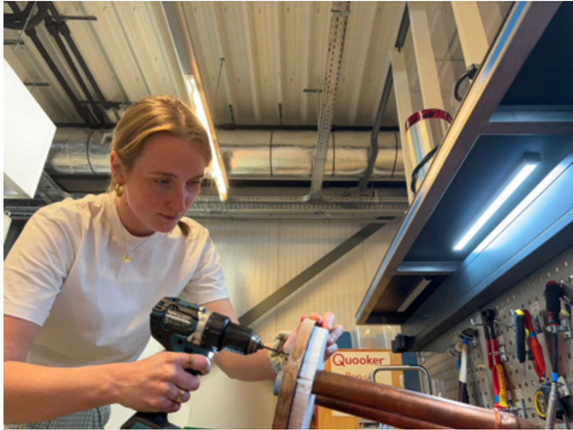
Drilling 10 mm holes for the cold water inlet and outlet of the buffer reservoir.
