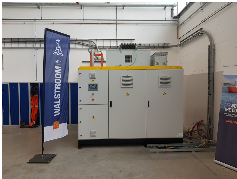
Figure 4.1: Picture of the shore power converter owned by Royal Roos
