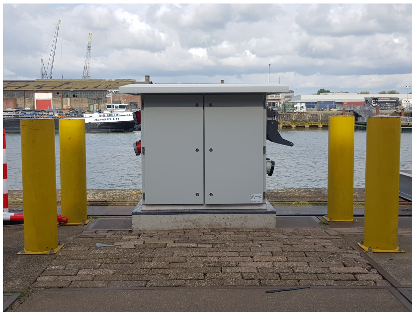
Figure 4.2: Picture of the shore power connection box owned by Royal Roos
