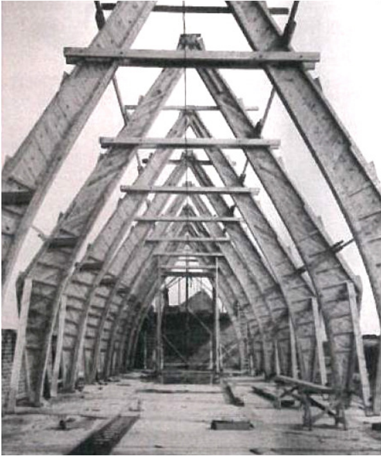
Image 1: Photograph from the construction of Diemerood work institute showing the boat like construction. Source: Het Nieuwe Instituut [photographer unknown]
