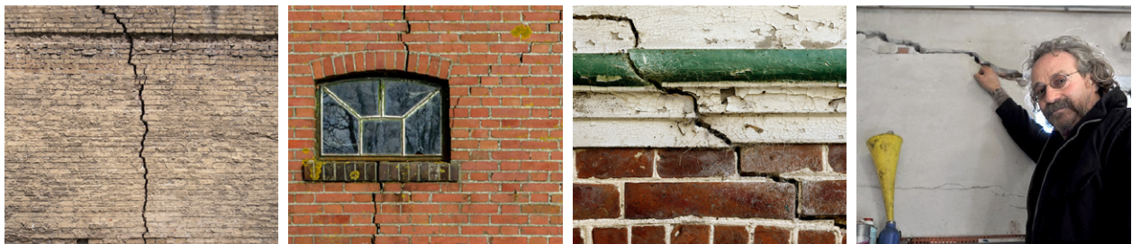
Figure 15: Damage on brick buildings in Groningen.
