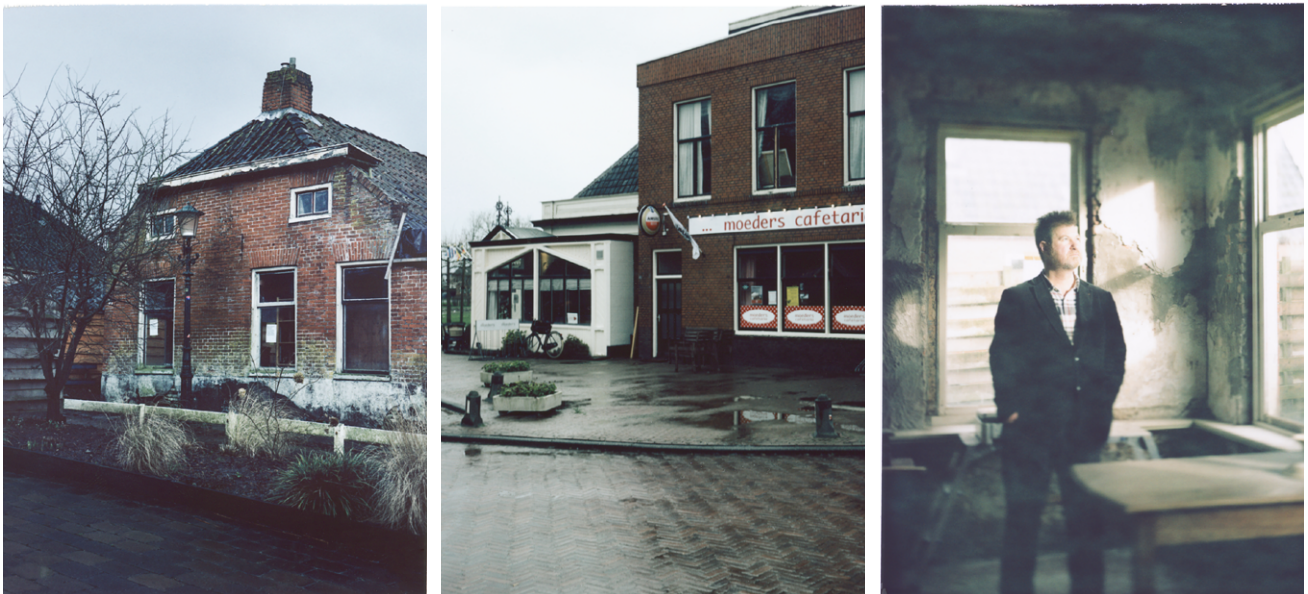
Figure 10: Earthquake damages in Warffum.
