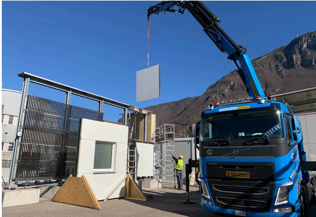
FIG. 3 Prefabricated façade elements were disassembled and transported to a shed to separate materials, to realistically emulate an end-of-life scenario.
