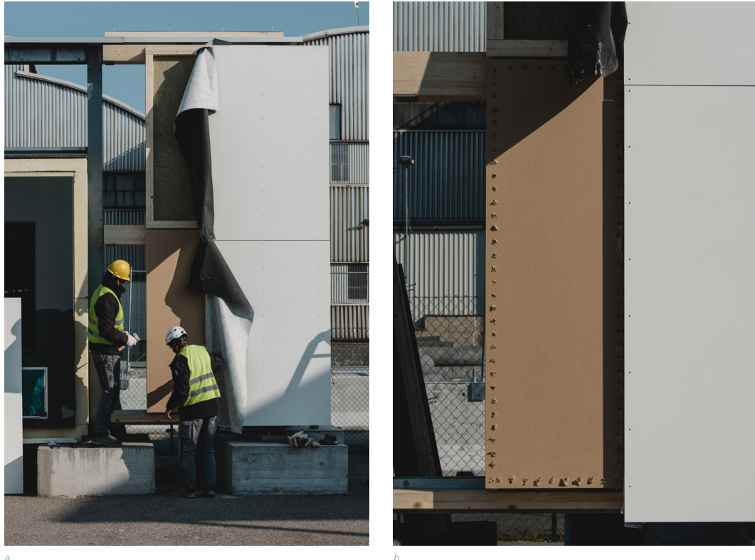
FIG. 2 Experimental activity to test the replacement of a façade layer. Image by Fiorentino.
