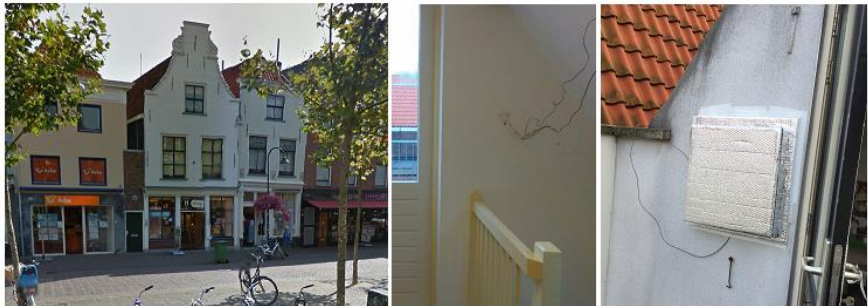
Fig. 2 Case study - The whole building (left), the inside surface of the wall (middle), and the outside surface and sensors covered by the box (right). Delft, Nov 2014
