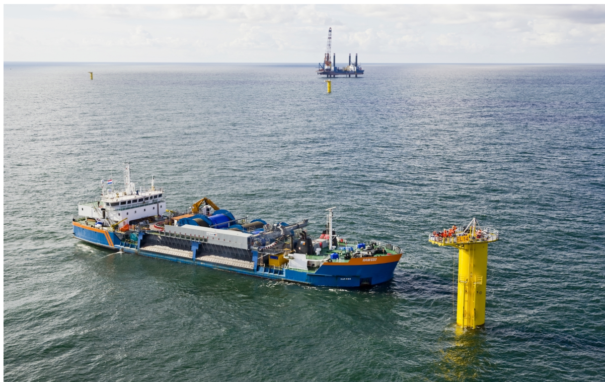
Figure 1.1: HAM 602 laying the infield cables at Gemini, Aeolus is installing monopiles in the background. (Van Oord, 2015)
