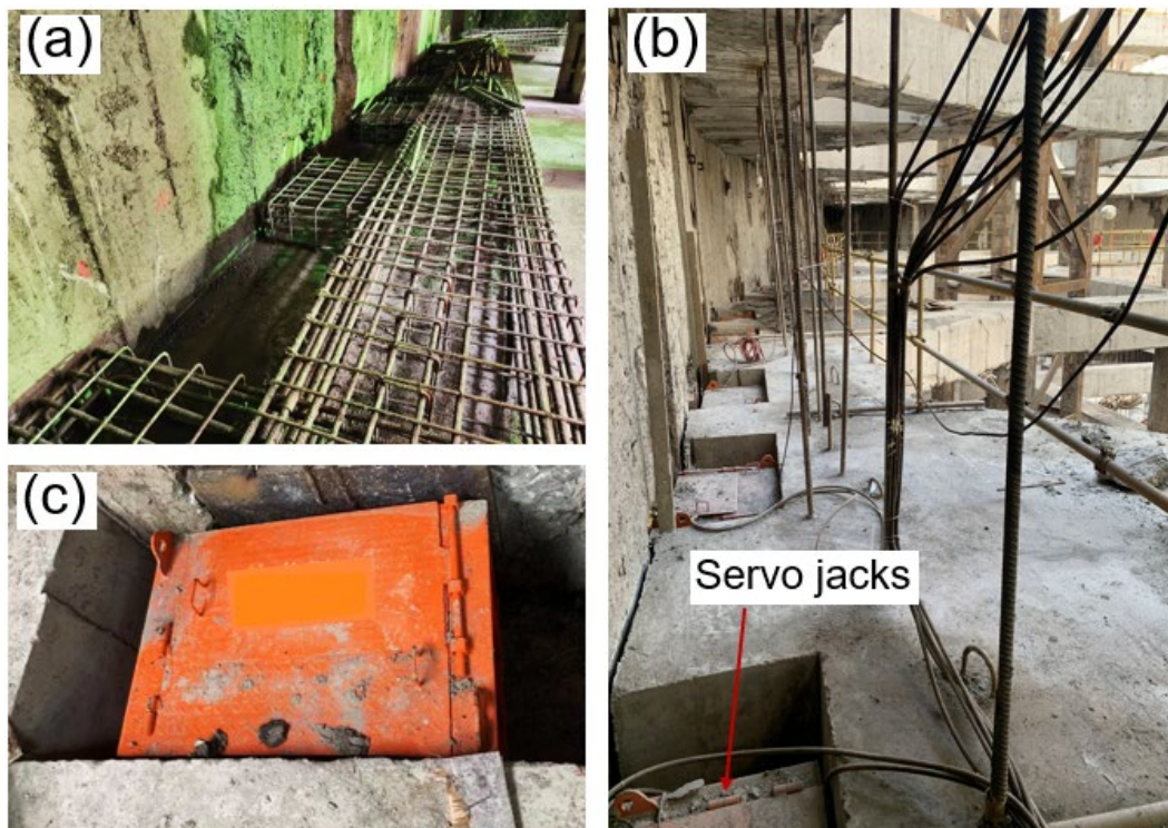
Figure 6. Bracing structure design of the Z3 with servo concrete struts: (a) reinforcement cage of purlin; (b) field construction of servo RC struts; and (c) servo-hydraulic jack.
