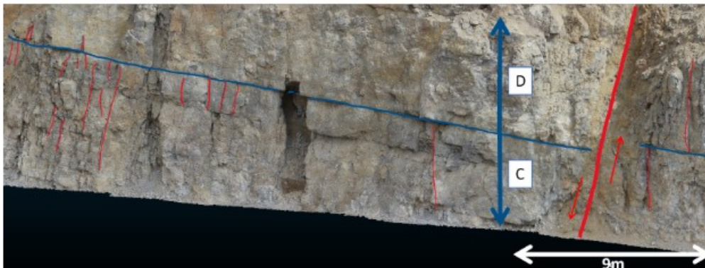
Figure 5.10: Bedding plane F delimiting formation D and C. Most joints are bounded by this bedding surface. A fracture swarm, or corridors can also be observed on the left of the figure.
