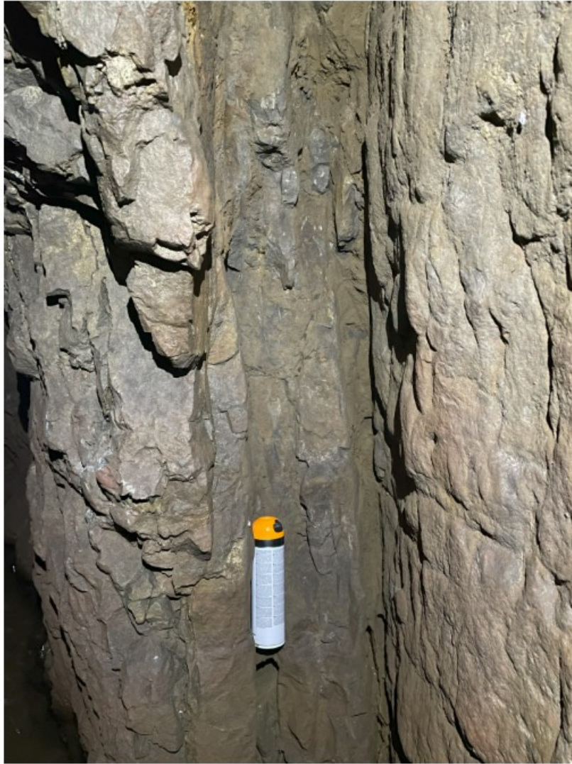
Figure 5.21: Structural joint with thick gouge infill.
