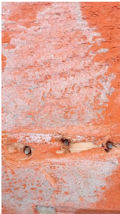
RUSTY SCREWS STUCK INSIDE THE FIBERS
