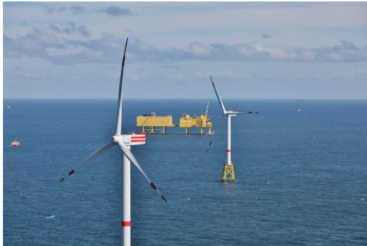
Figure 2. TenneT / HelWin alpha Offshore HVDC substation (picture taken from [4]).
