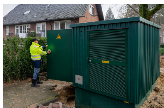
(b) 'Middenspanningsruimte' (MSR) acting as network node by connecting underground cables on the medium-voltage distribution grid. (As seen in a residential area)
