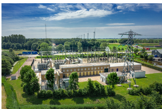
(a) Substation that transforms high-voltage power from the transport grid to medium-voltage power to be distributed on the distribution grid. (Onderstation Bolsward)
