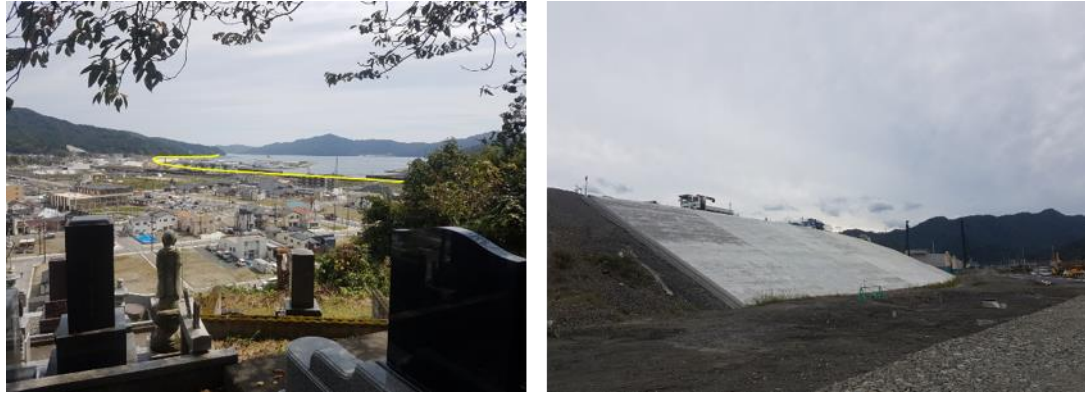
Figure 2: Left: Otsuchi Town (Sanriku coast), the yellow line indicates the location of the planned sea dyke. Right: Sea dyke under construction, height is 14.5 m. Photos: (Roubos 2018)
