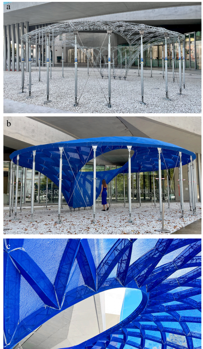
Fig. 19. KnitNervi demonstrator at MAXXI, Rome (a) at the stage of the completed double-layered gridshell structure that serves as falsework and reinforcement, (b) with the knitted shuttering from an external perspective and (c) as an internal closeup with oculus and prismatic sections with rebar cages inside.
