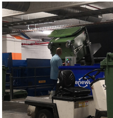
28. The waste from the containers is pressed together and then incinerated.
