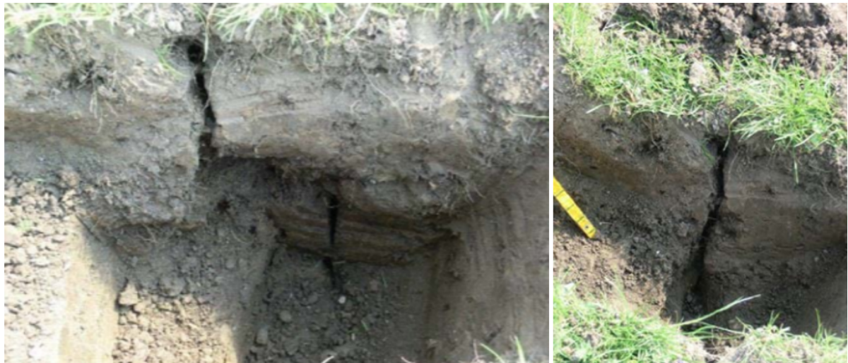
Figure 2.15: Cracks in Dutch clay dykes, observed in 2013 (Alterra, 2013)
