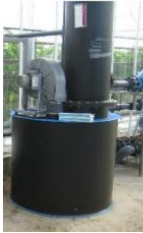
Figure 4. 20 Reservoir of tower aerator
