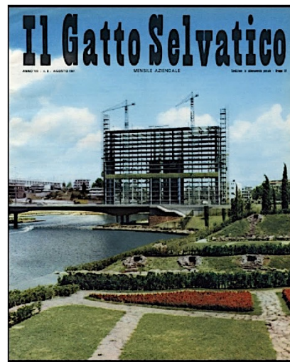
Figure 9. The powerful and agile structure of the new E.N.I Palace at EUR in advanced construction phase. Romano Costa. The powerful and agile structure of the new E.N.I Palace at EUR in advanced construction phase . Rome: Il Gatto Selvatico 1961 (Year VII), August, n°8. A4 Photograph. ENI Archive, Castel Gandolfo, accessed March 5, 2020.
