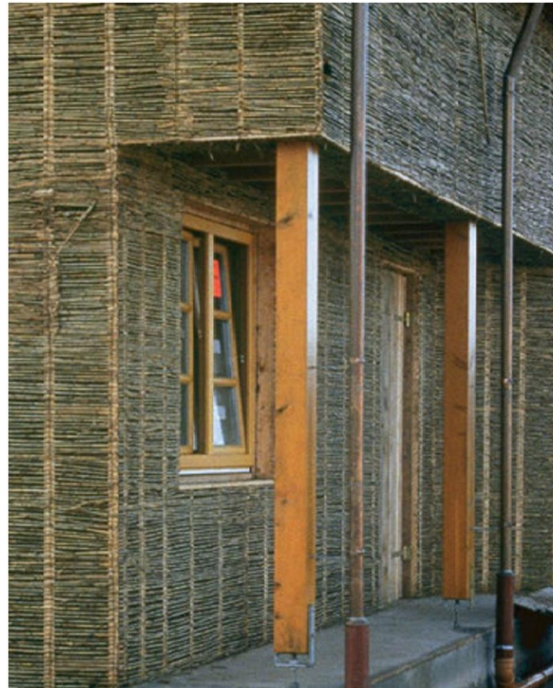
Figure 4. Lost formwork for woodchip light earth using reed plaster lath. From Light Earth Building (p. 94), by Volhard, F., 2016, Birkhäuser.
