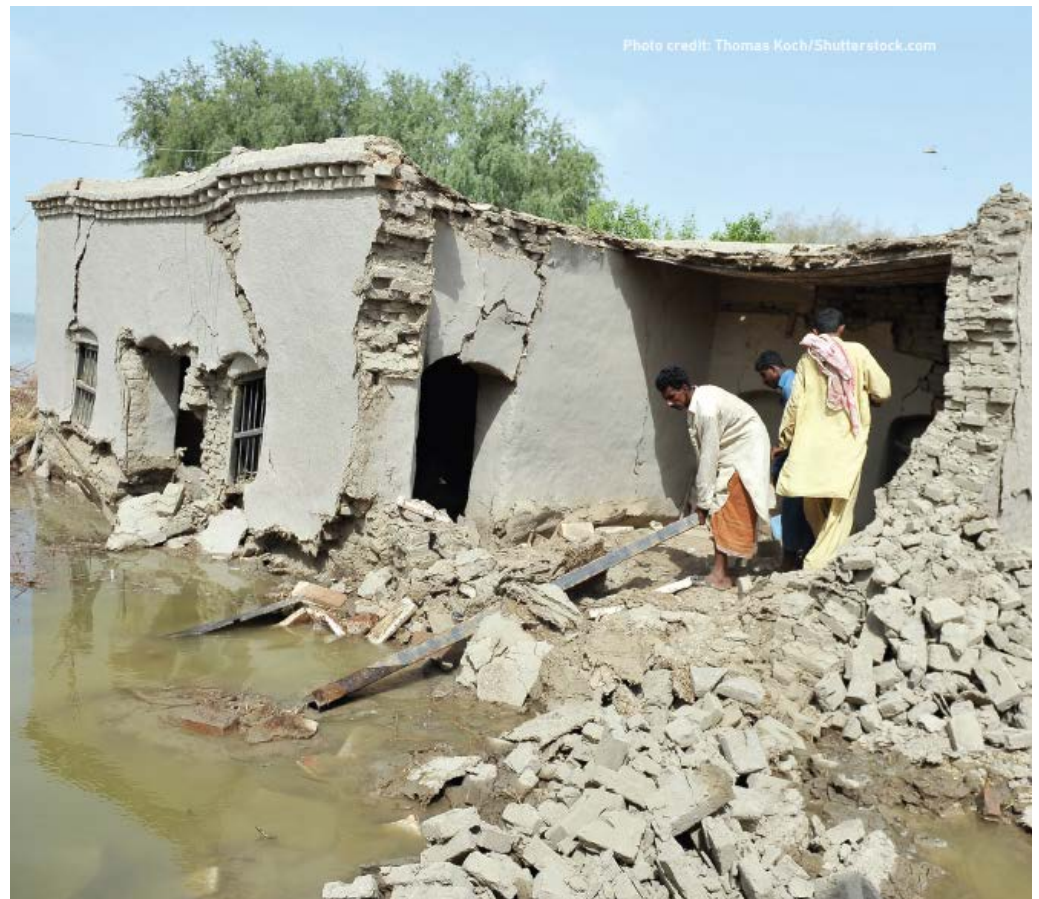
Figure 53. Flood damage; Photo: Thomas Koch / Shutterstock.com
