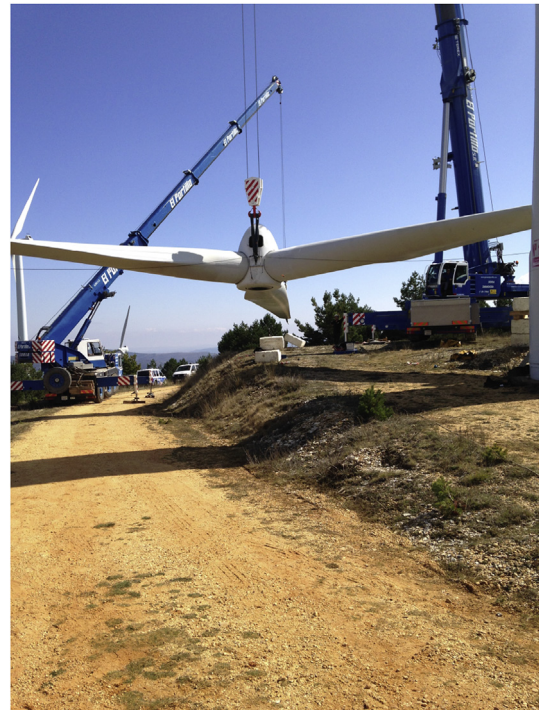
Fig. 3. Photograph of a blade replacement in the wind farm investigated (copyright, CETASA).
