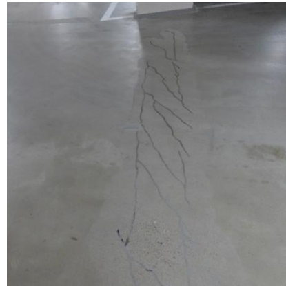
Figure 5.2: Cracks along the support of slab element (Adviesbureau Hageman).
