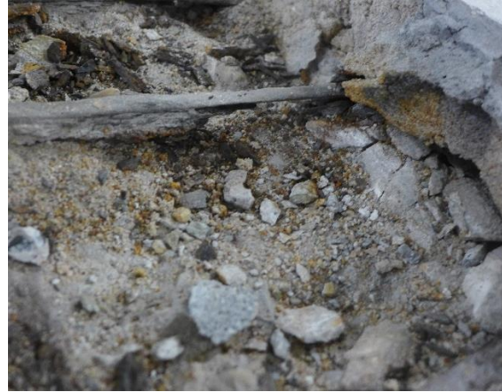
Figure 5.6 Corrosion of reinforcement in compressive layer (Adviesbureau Hageman).
