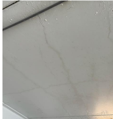
Figure 5.20 Cracking at underside of filigree slab (Adviesbureau Hageman).
