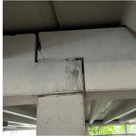
Figure 5.30 Local support end failure of half-joints (Adviesbureau Hageman).
