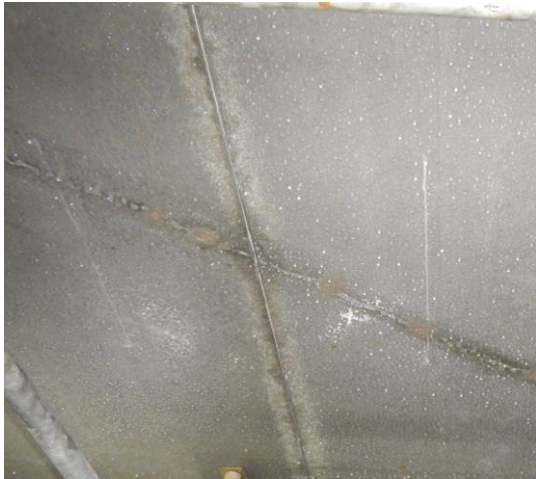
Figure 5.19 Cracks running through adjacent filigree slab elements as result of restrained deformations (Adviesbureau Hageman).
