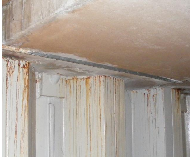
Figure 5.46 Leakage at connection between sheet pile wall and concrete floor (Adviesbureau Hageman).
