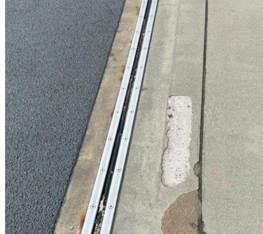
Figure 5.48 Cracking next to expansion joint due to incorrect installation (Adviesbureau Hageman).
