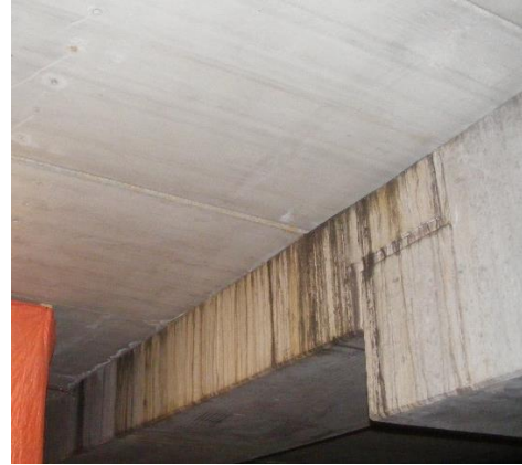
Figure 5.10 Leakage at support joint of hollowcore slab (Adviesbureau Hageman).
