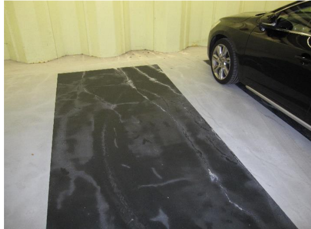
Figure 5.26 Cracks along connection between sheet pile wall (Adviesbureau Hageman).
