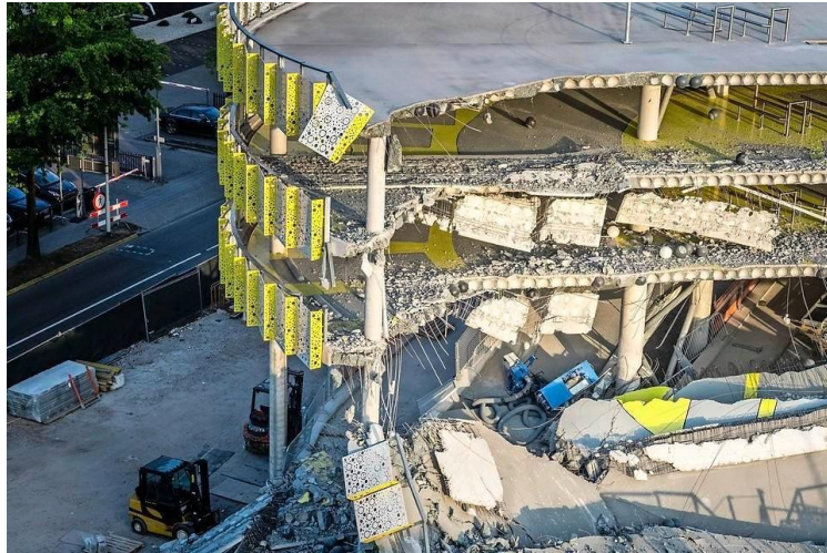
Figure 5.17: Collapse of parking garage using filigree floors (Engelaar, n.d.)
