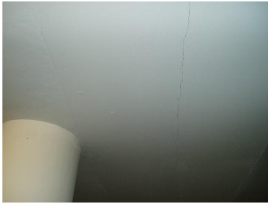
Figure 5.13 Cracks at the underside of hollowcore slab (Adviesbureau Hageman).
