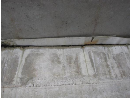
Figure 5.33 Extruding elastomeric bearing pads at support of slabs (Adviesbureau Hageman).
