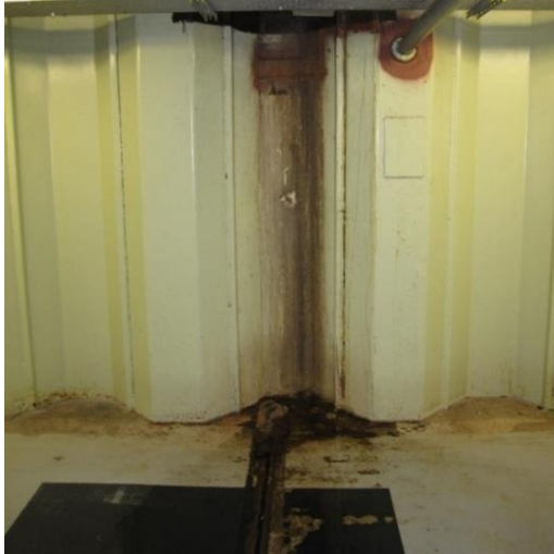
Figure 5.45 Leakage at sheet pile wall located at floor joint (Adviesbureau Hageman).
