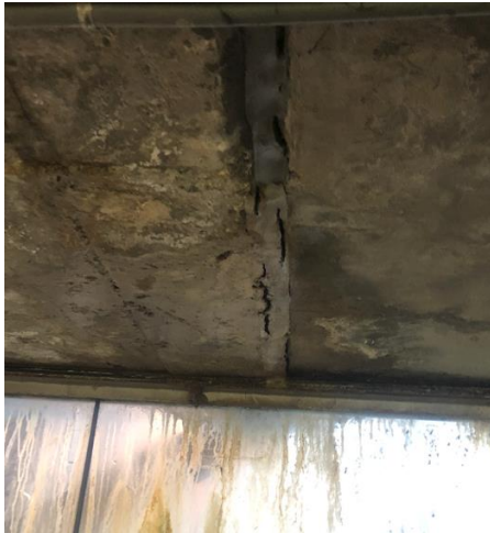
Figure 5.51 Failure of adhesion and leakage of joint (Adviesbureau Hageman).
