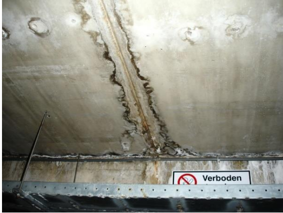
Figure 5.9 Leakage at longitudinal joint of hollowcore slab (Adviesbureau Hageman).
