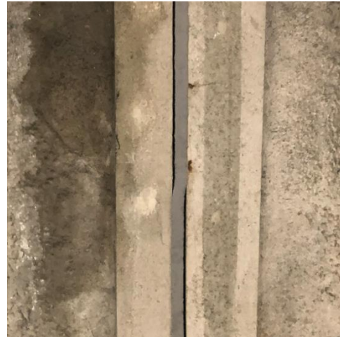
Figure 5.52 Adhesion failure of joint sealant (Adviesbureau Hageman).
