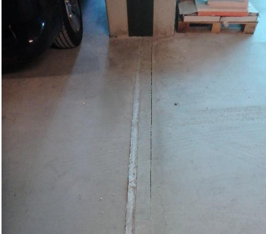
Figure 5.47 Cracking beside expansion joint (Adviesbureau Hageman).
