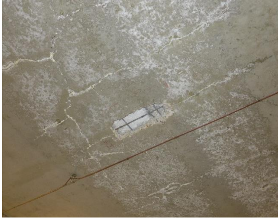
Figure 5.5 Cracks as result of corroded rebar (Adviesbureau Hageman).
