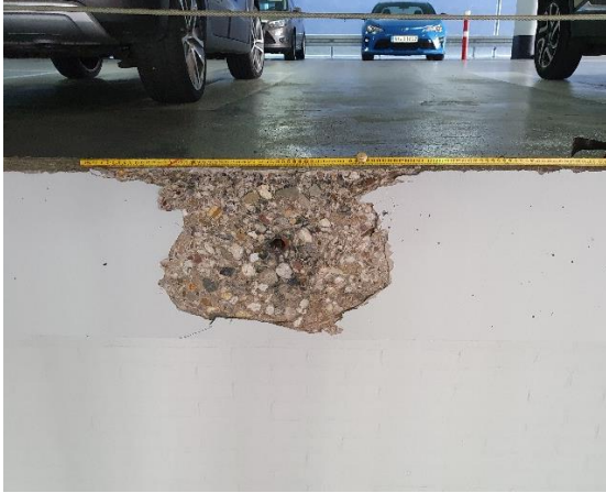
Figure 5.23 Spalling as result of failure of prestress tendon (Adviesbureau Hageman).
