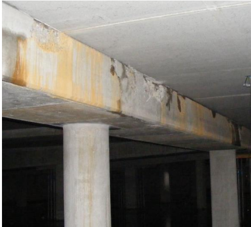
Figure 5.29 Local support end failure of concrete support beam (Adviesbureau Hageman).
