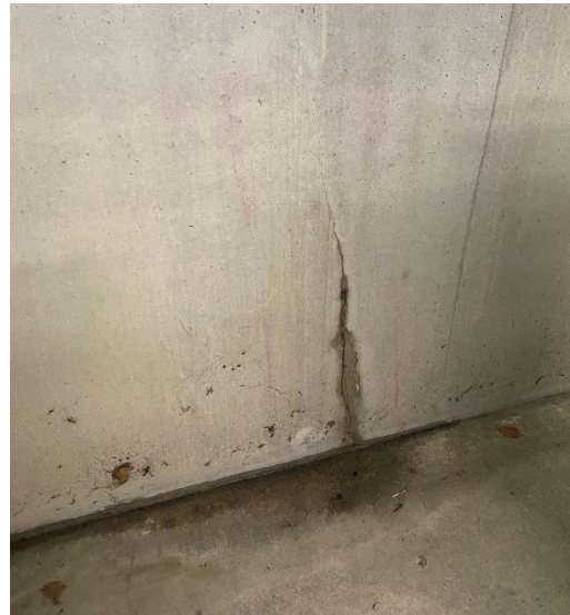
Figure 5.40 Cracking in concrete cast in-situ wall, increasing in crack width towards the floor element (Adviesbureau Hageman).
