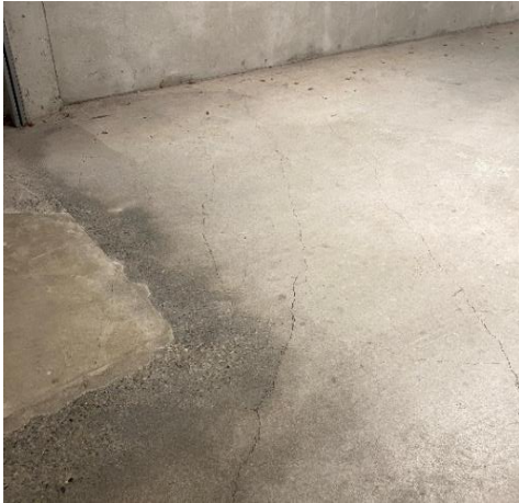
Figure 5.25 Cracks in monolithic floor, restraint by adhering walls (Adviesbureau Hageman).
