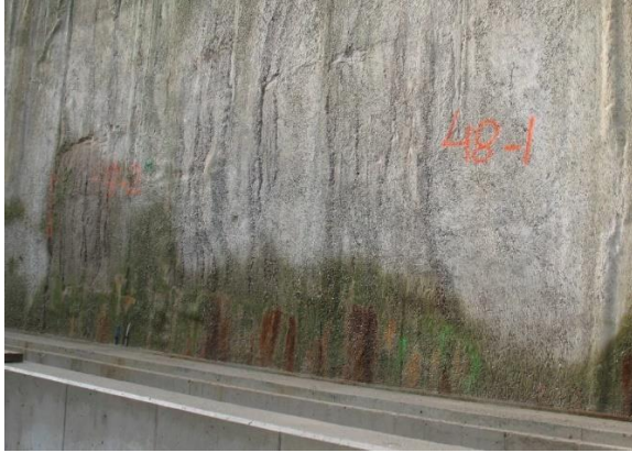
Figure 5.42 Leakage right above concrete beam element (Adviesbureau Hageman).
