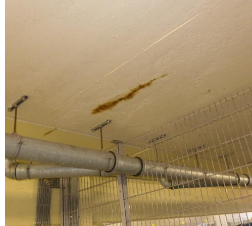
Figure 5.24 Visible exposed tendon lubricant (Adviesbureau Hageman).
