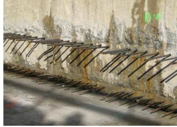
Figure 5.43 Leakage at protruding bars in diaphragm wall (Adviesbureau Hageman).
