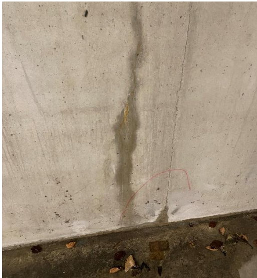
Figure 5.39 Cracks in cast-in situ wall, accommodated by leakage (Adviesbureau Hageman).
