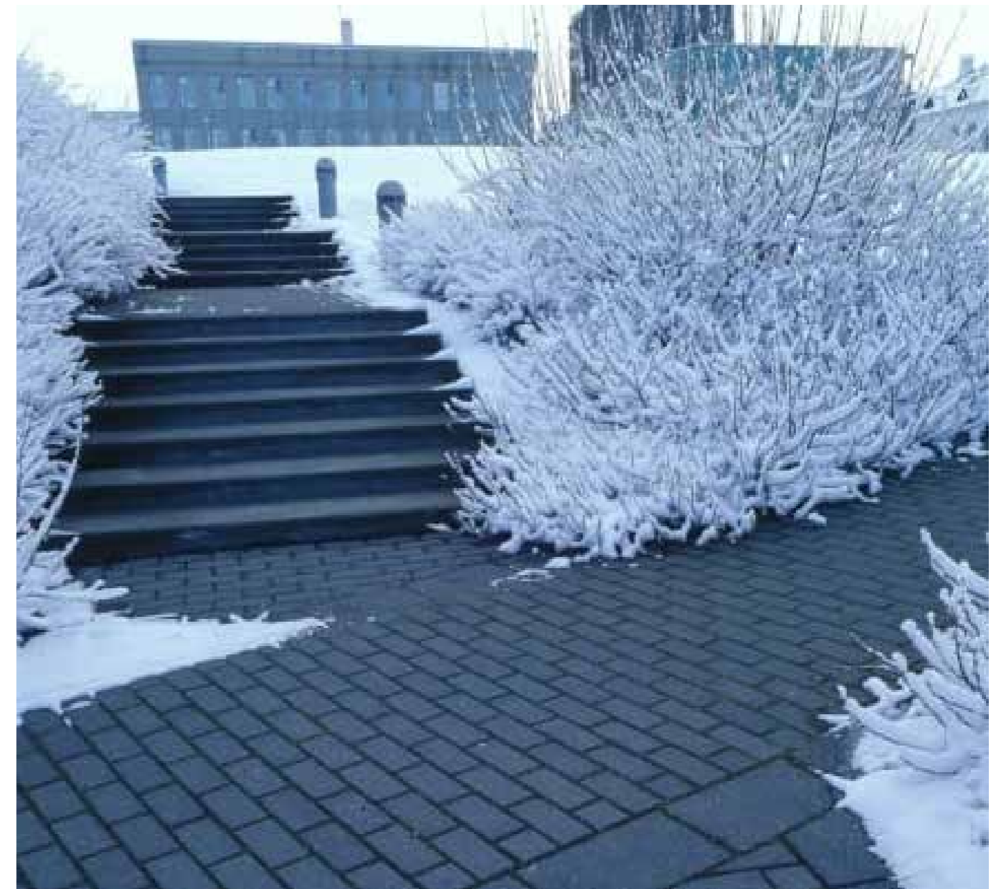
Figure 143 Sidewalk Iceland District Heating System. Source: Heated Sidewalks: Iceland has them, Saskatoon Wants Them, CBC.
